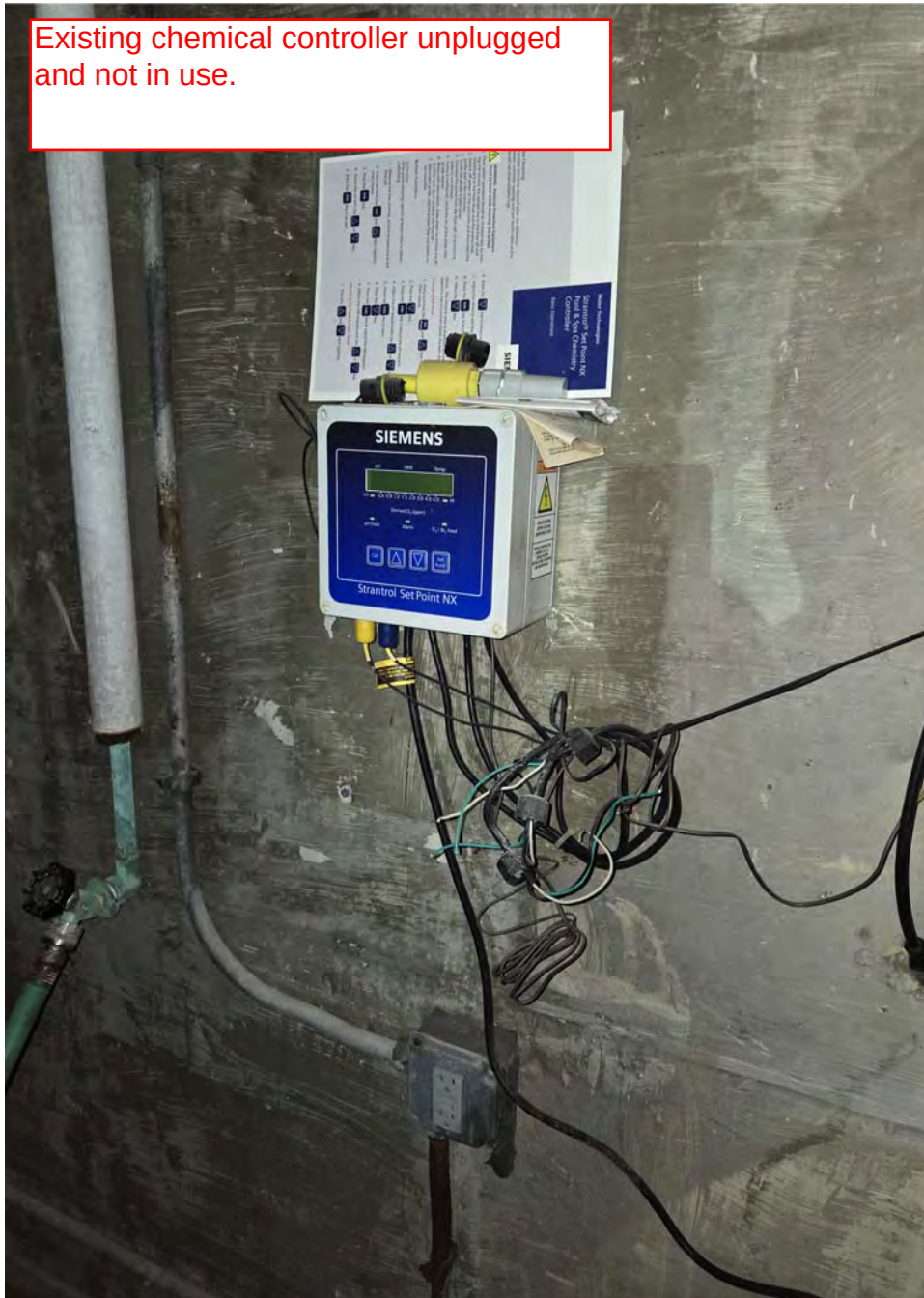
Flow cell for existing chemical controller
